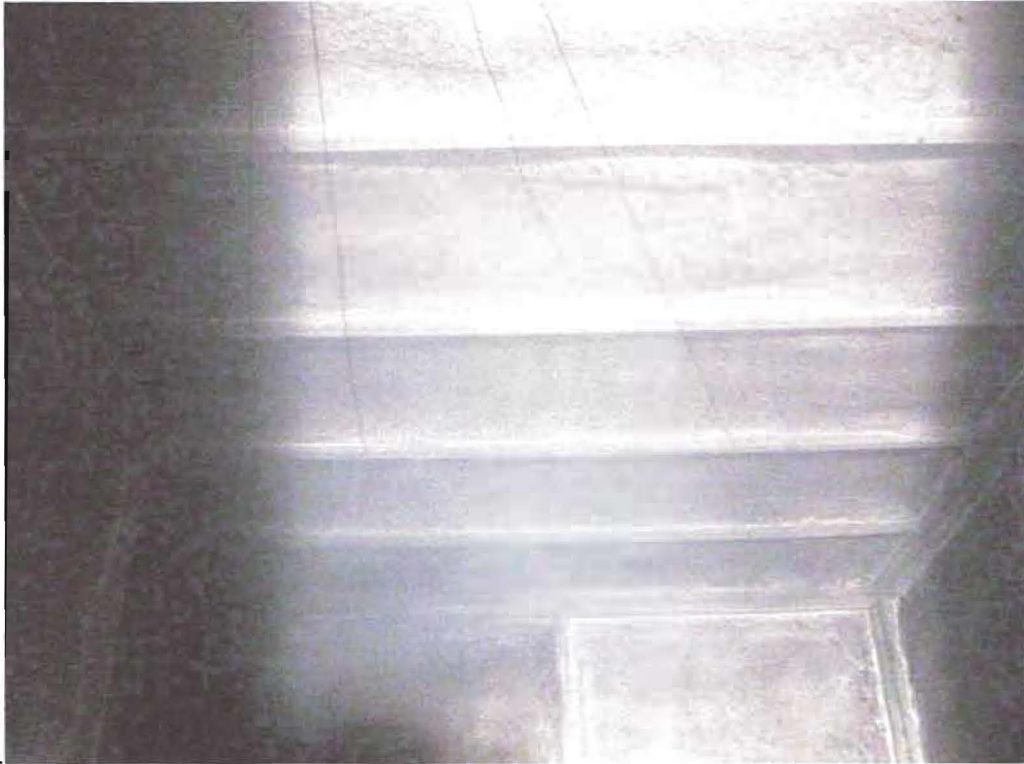
Post-test photo of ceiling
