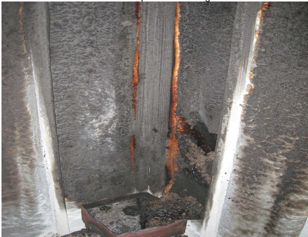
Post-test photo corner above burner
